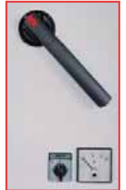
Individual Circuit Monitoring
